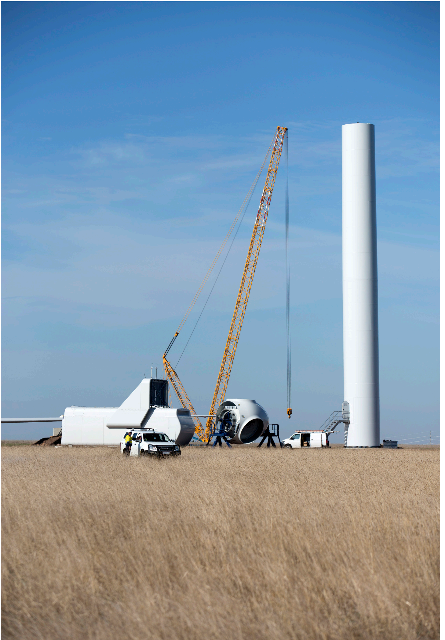
Salt Creek wind farm, Victoria
