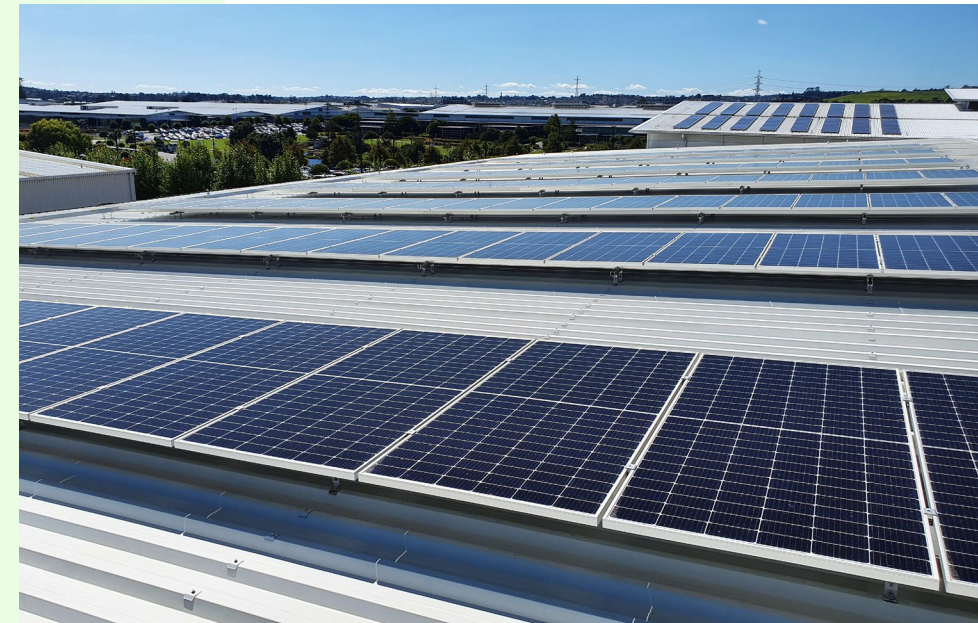
PMA, Highbrook Business Park, solar panels installed on existing property
